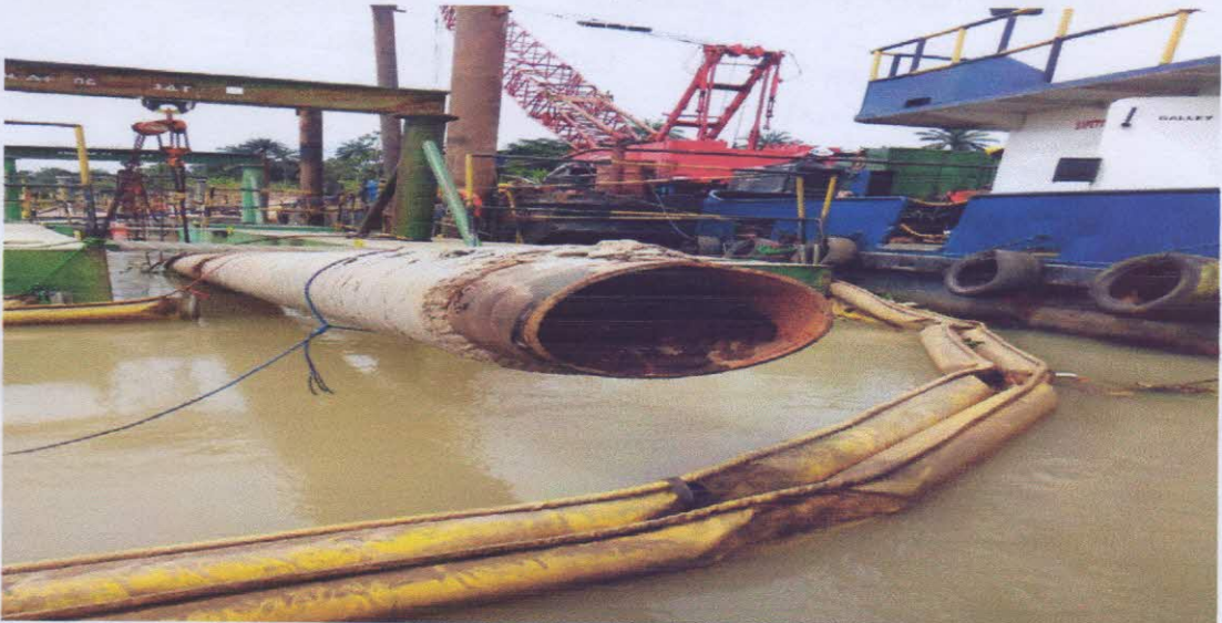
Below is picture showing the bron the broken pipeline and the floater with which it was lifted.
